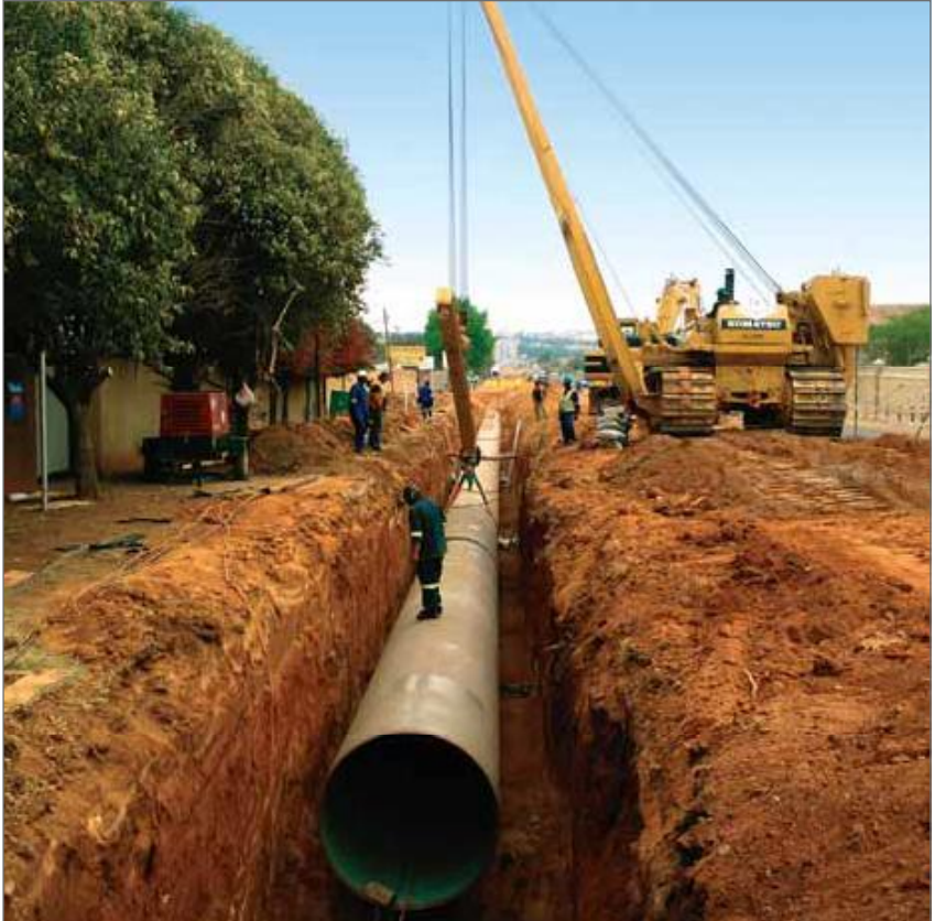
M&D Construction has the expertise and equipment to undertake the laying of large-diameter steel water pipelines – here a 1 700 mm diameter steel pipe is being positioned on the Rand Water Q5 contract
